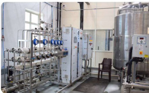
WATER PURIFICATION SYSTEM
