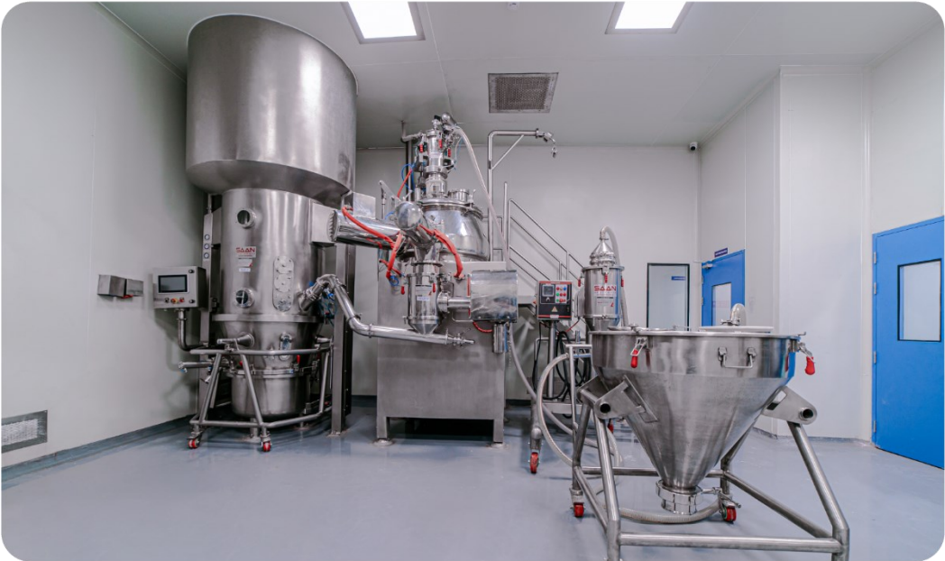
Integrated Granulation Line (Vacuum transfer system with LPD)
